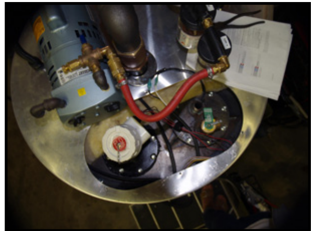
TOP OF USED COOKING OIL TANK
